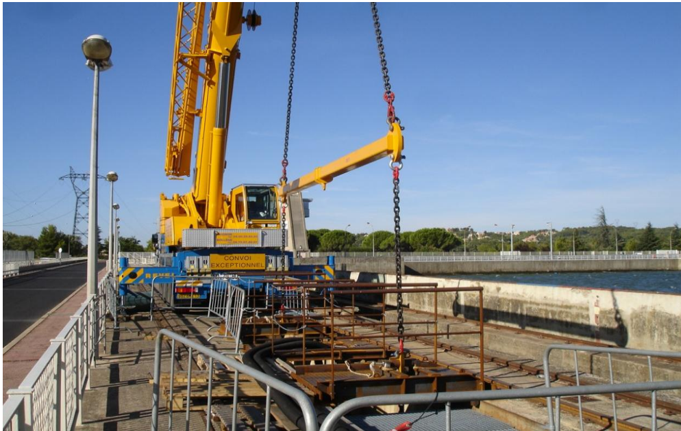
Figure 2-1 Crane positioning fish release pipes into the intake gate slot of Turbine Unit 3 at Beaucaire Power Station.
